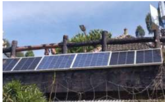
Figure 4. 2 Posong Solar Panel System
