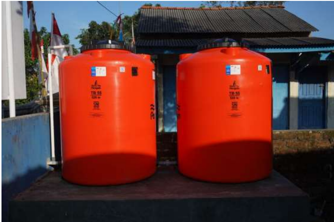
Figure 2. Clean Water Reservoir
